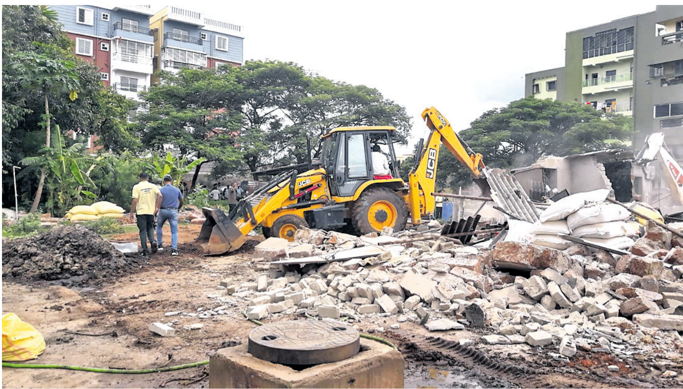
EVICTON DRIVE: An excavator deployed by BDA razing down unauthorised constructions in Patia area of Bhubaneswar, Thursday
