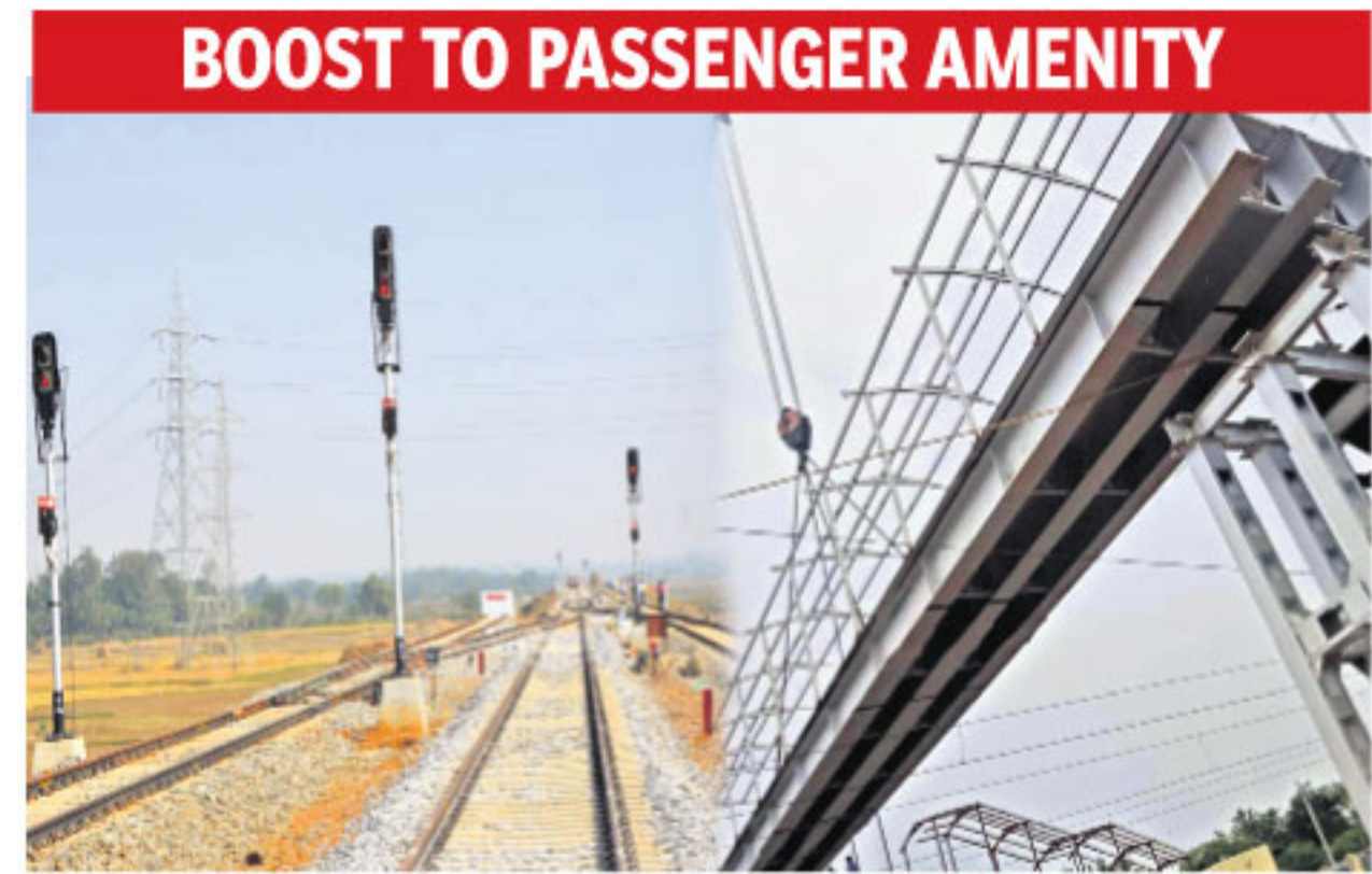
18 LHSs have been completed at various places, including closure of three manned level crossings by providing alternate ways
