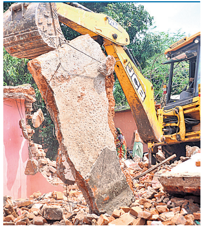
Buildings of Behera Colony at SCB Medical College and Hospital in Cuttack being demolished for expansion of the state-run health institute, Tuesday
