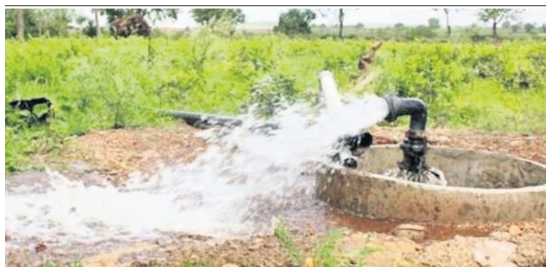
Now the focus is on Golamunda block of the district. The block is comparatively less irrigated than other parts. Five new minor irrigation projects will be set up in the block. It was also learnt that the government has decided to restore 13 irrigation projects in the district
