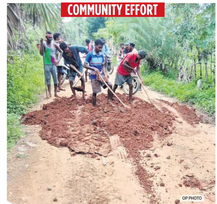
Villagers repair the road from Koyaguda to Canal Bank road under Korukunda block in Malkangiri. The road work allegedly botched up by a contractor
