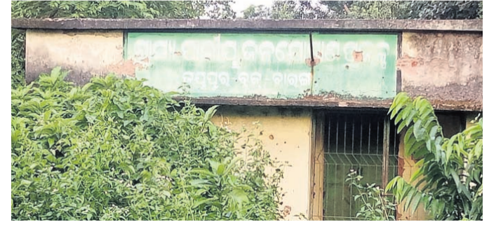
lakh to sink a borewell, build a pump house and lay pipes for the drinking water project. However, the project is yet to be made functional even though 15 years have passed since its construction.
