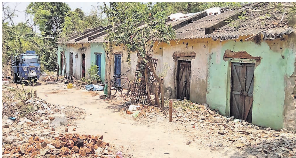
Damaged houses of the Yugoslavia Colony in Paradip.
