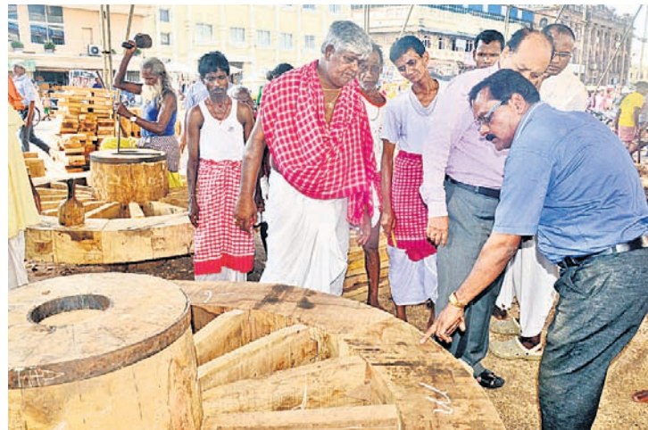
Investigating team checking the defects in the chariot wheel at Rathayard, Puri
