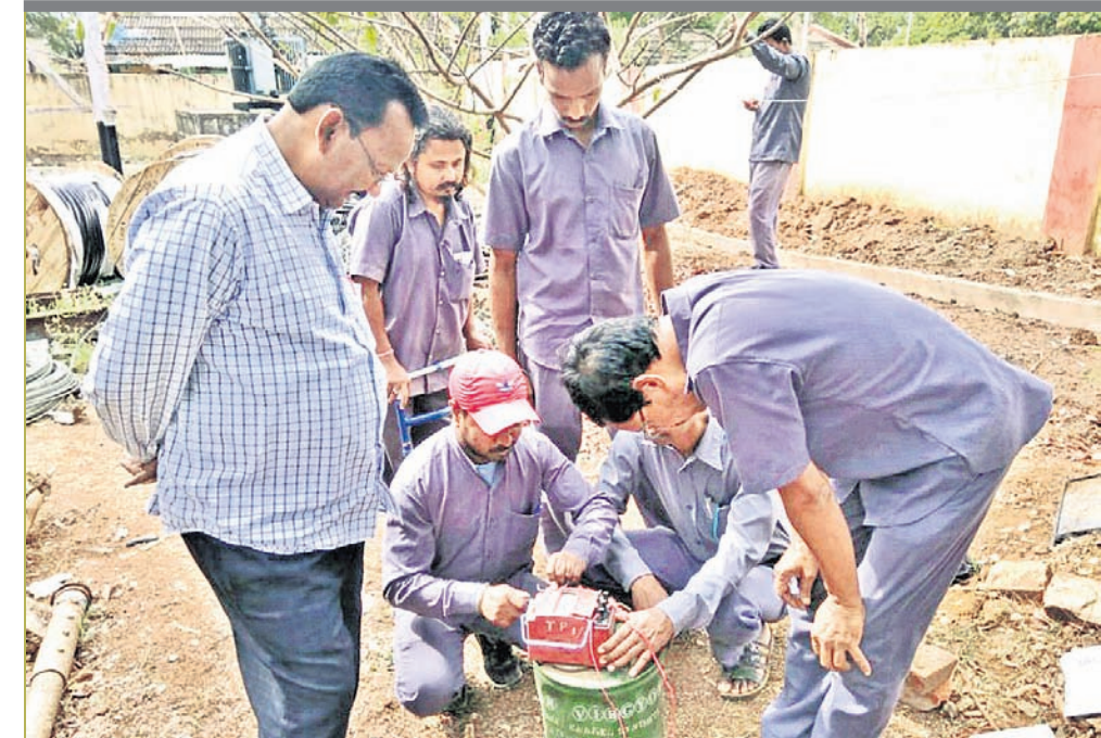
Railway officials conducting an earthing test as part of electricity safety week in Sambalpur Tuesday. OP PHOTO
