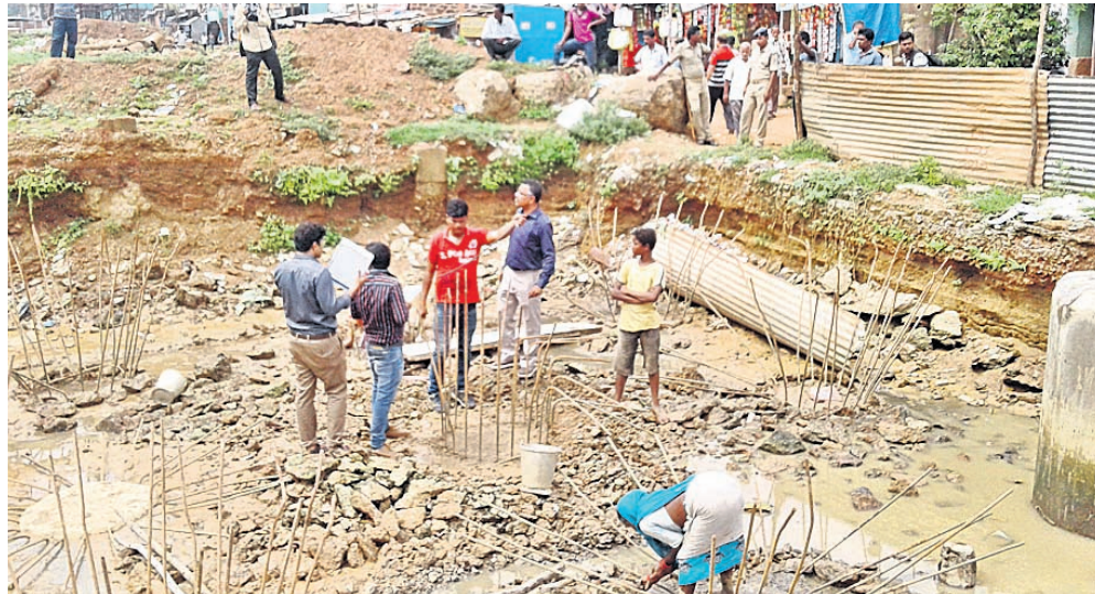
An NIT team inspecting the project site at Jatni (A file photo)
