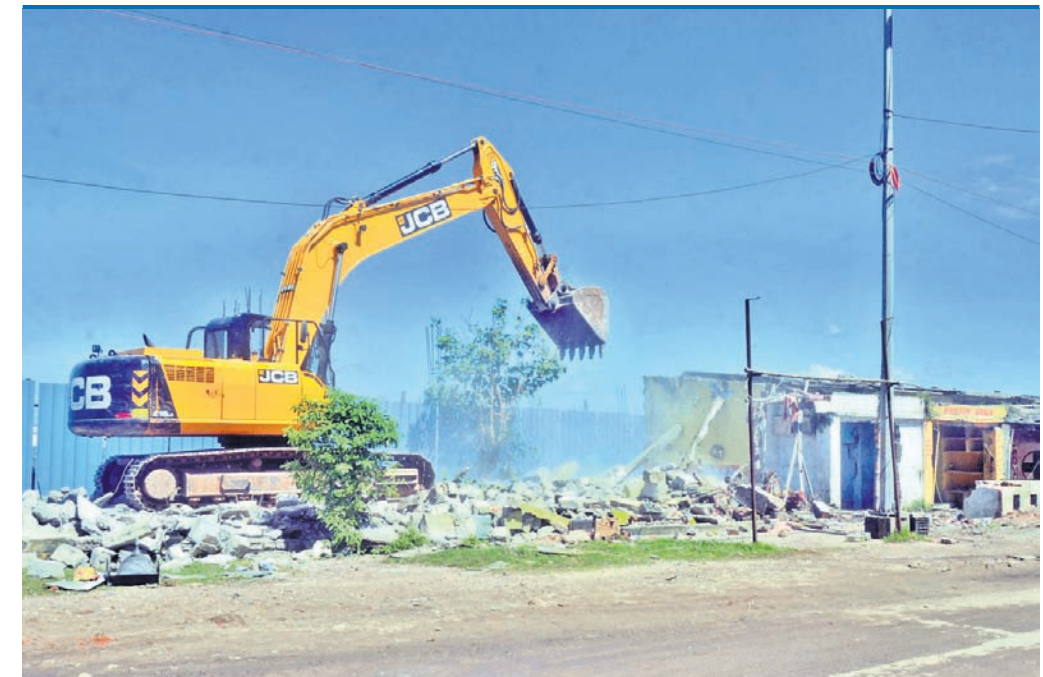
An excavator engaged by the civic body pulls down dilapidated shops at Penthakata in Puri, Tuesday
