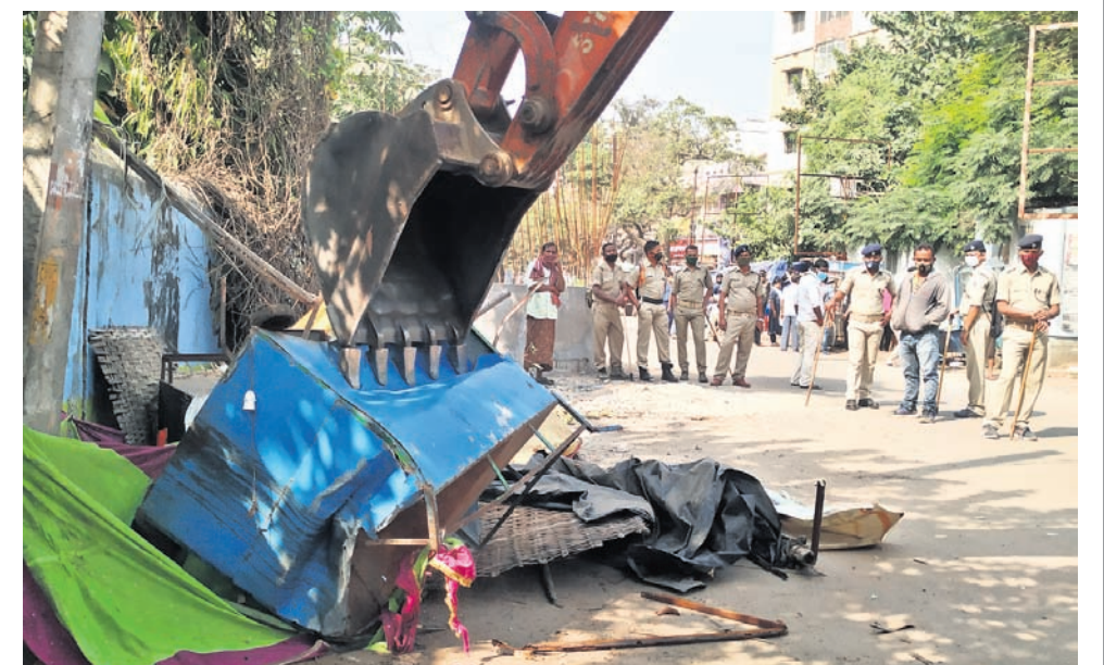
An excavator engaged by Cuttack Municipal Corporation pulls down illegal structures between the railway station and College Square in the Silver City, Monday (OP PHOTO)
