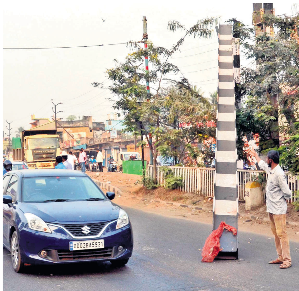
Damaged height restriction bars near Madhupatna Railway Bridge in Cuttack pose threat to the commuters OP PHOTO
