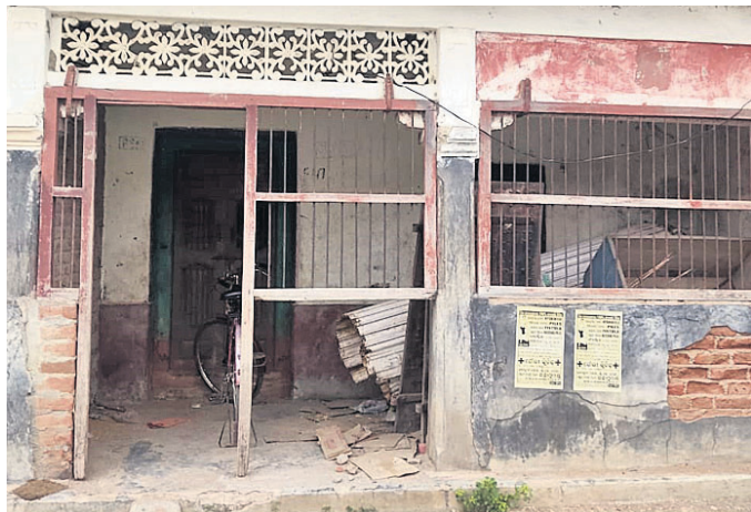
A house lies abandoned by its occupants in Patrapur area
