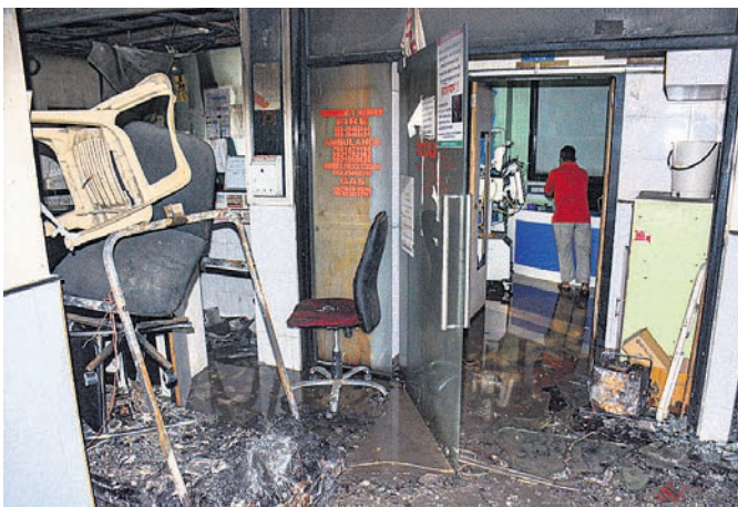
A section of the Prime Criticare Hospital in Thane which was razed to ashes due to the flames Wednesday
