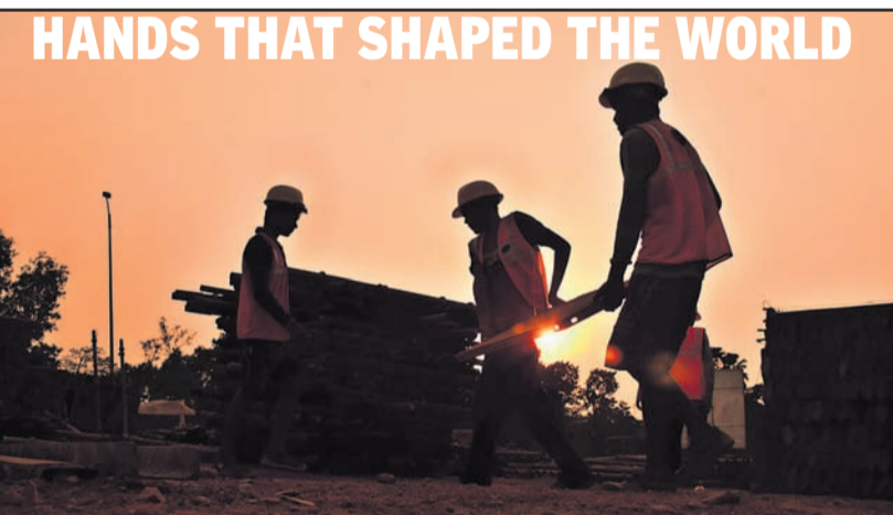
Workers engaged at a construction site near Nayapalli in Bhubaneswar, Friday, even as the world celebrates International Labour Day, Saturday
