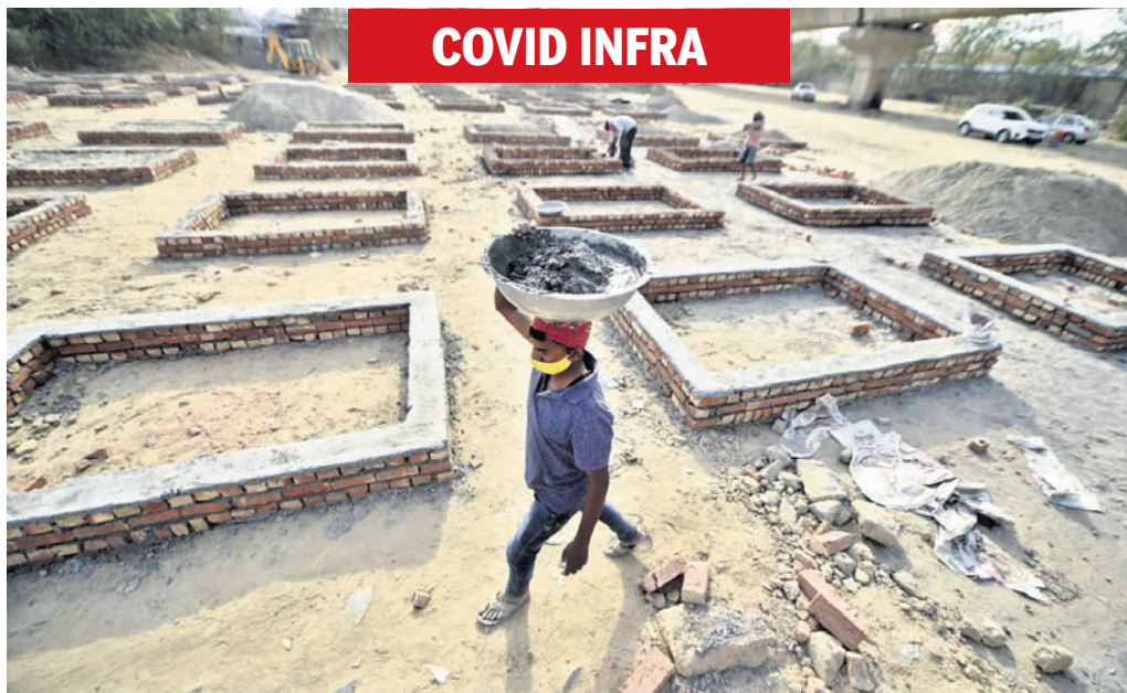
Workers build new platforms to cremate COVID-19 bodies, as coronavirus cases surge in record numbers, outside Sarai Kale Khan Crematorium in New Delhi, Friday
