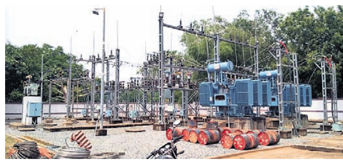
The project has crossed its deadline, which expired six months back, but work on the project is yet to be completed
