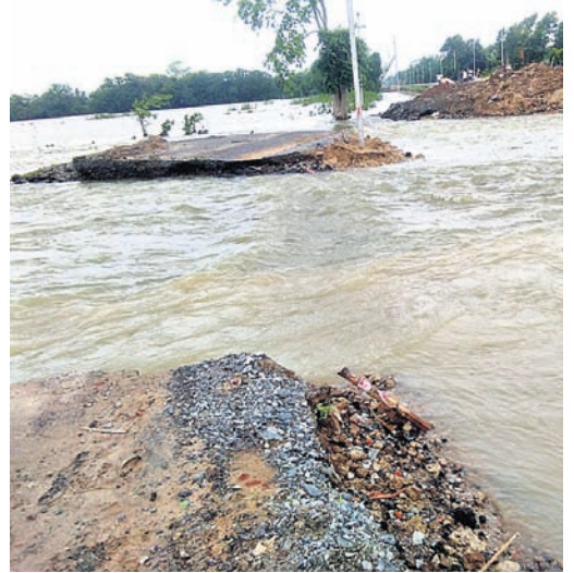
Rain water overflowing on Basudevpur- Jamujhadi road in Bhadrak following a breach
