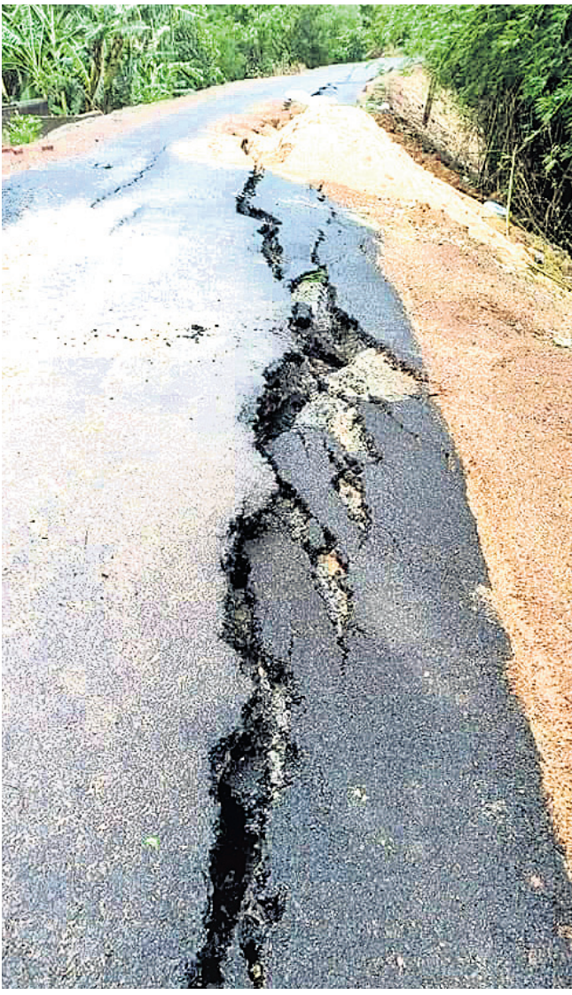
Cracks appear on a road in Dhamnagar block of Bhadrak
