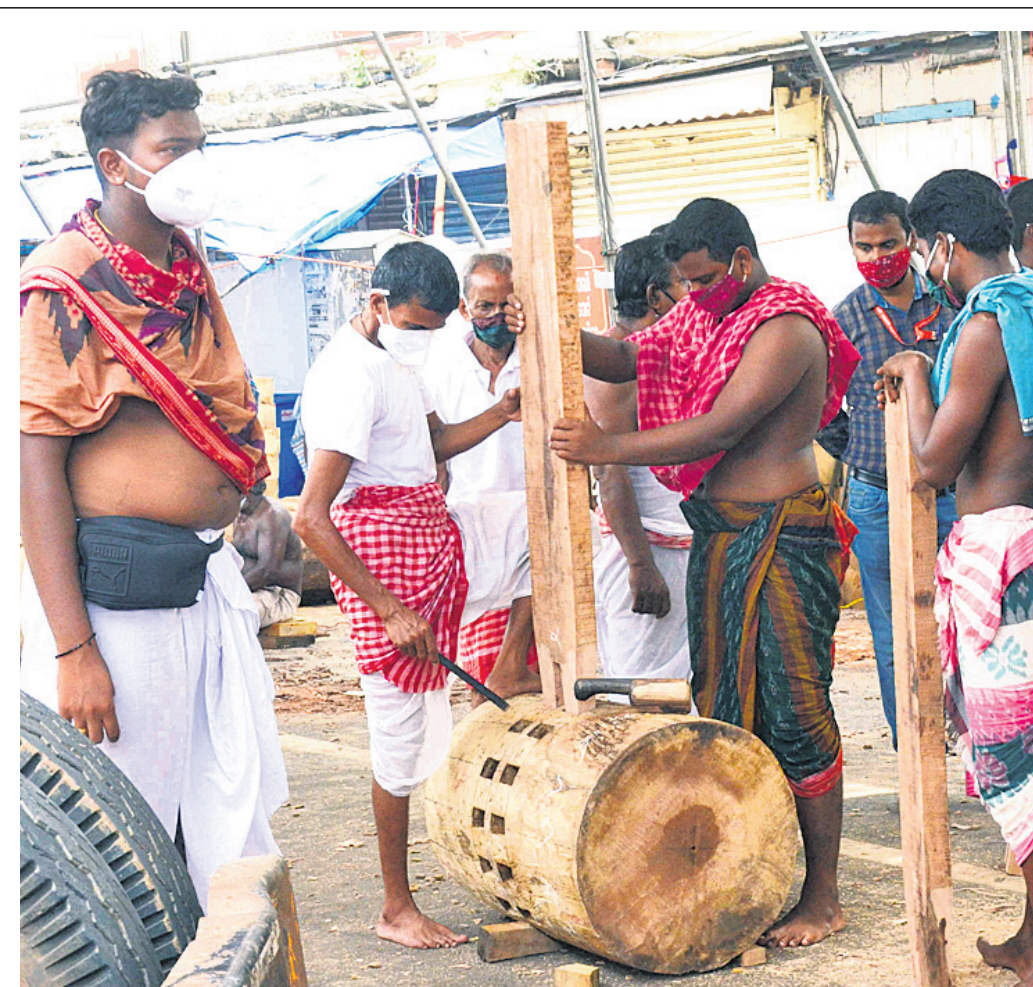
Carpenters fixing spokes to a hub as part of the chariot construction work at Rath Yard in Puri, Thursday
