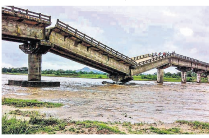
A bridge at river Kanchi collapsed due to heavy rain
