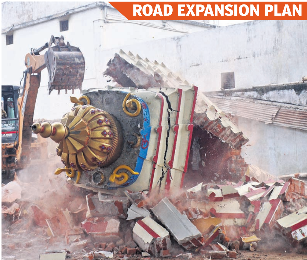
A temple being demolished at Telugu Sahi near Chhatra Bazar in Cuttack, Wednesday, to facilitate the expansion of Taladanda canal road
