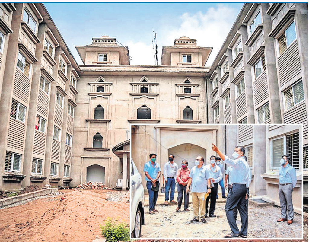
Srimandir chief administrator Krishan Kumar along with other officials (inset) inspects an under-construction shelter house for devotees in Puri, Wednesday
