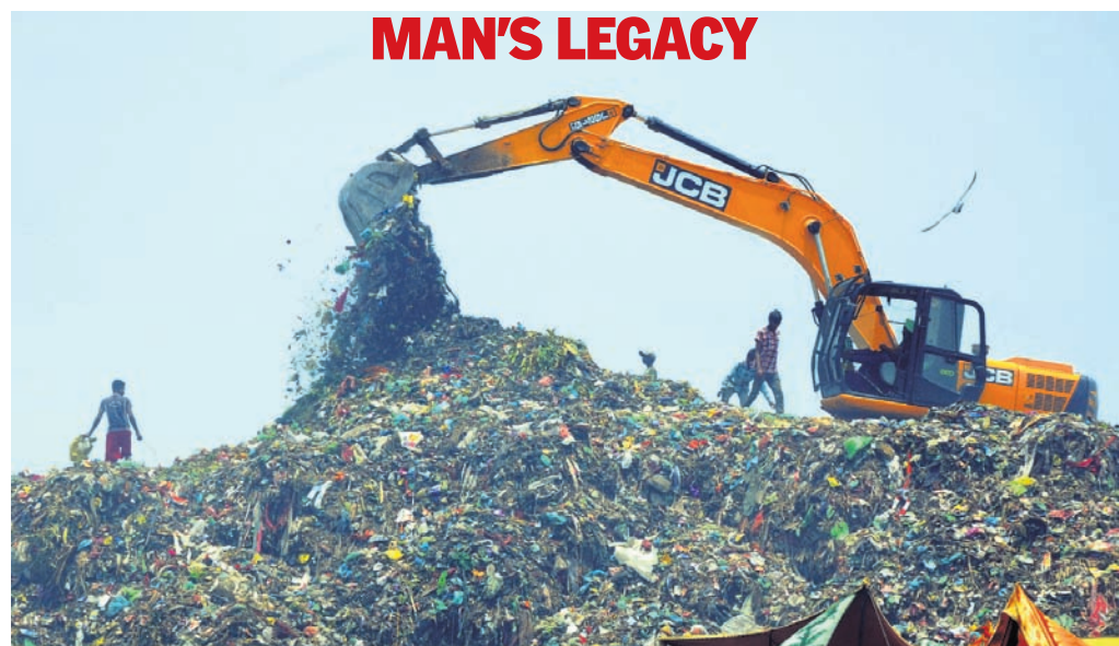
Crane operators busy at a garbage dumping ground on World Environment Day, in Amritsar, Saturday
