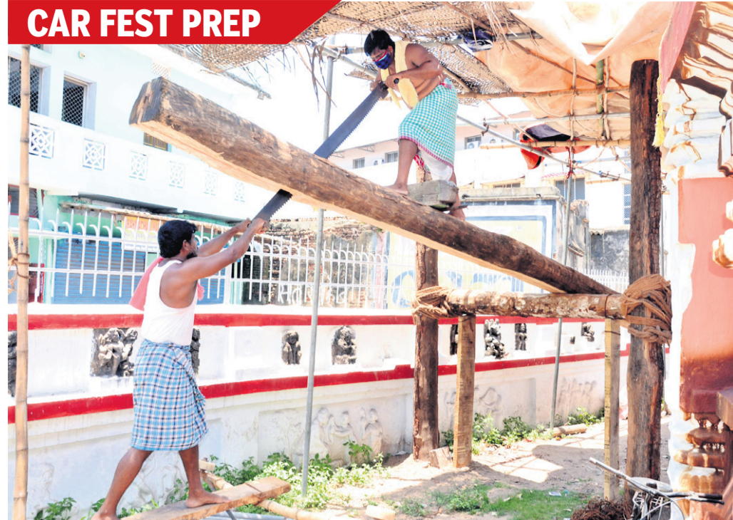
Chariot construction for the upcoming Rath Yatra in progress at Rath Yard in Puri, Sunday
