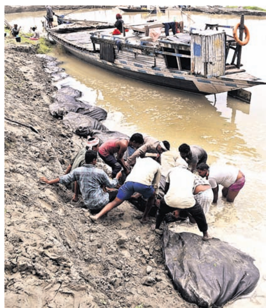
Workers put sandbags on the bank of the River Brahmaputra to control soil erosion ahead of the monsoon season in Guwahati, Tuesday
