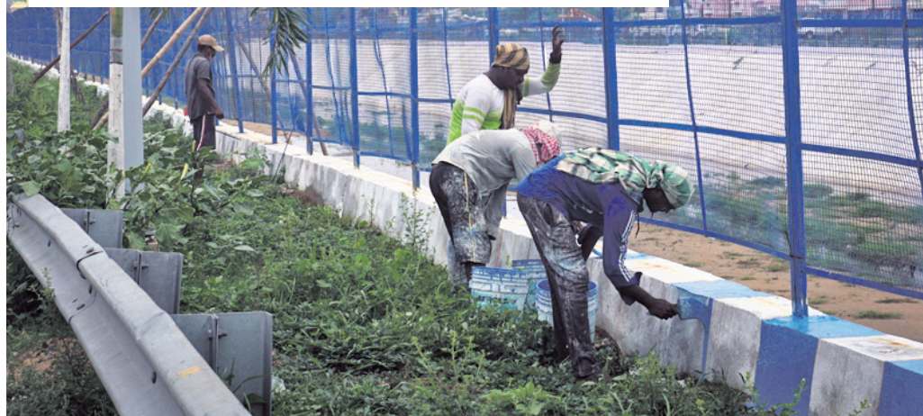
Work in progress for Taladanda canal (inset) renovation and beautification project in Cuttack, Saturday
