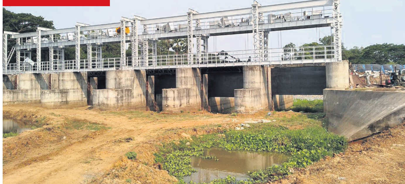
The Water Resources department has constructed a barrage on Prachi river at Kakatpur in Puri with an expenditure of ₹20 crore. The project will help in flood control and irrigation activities
