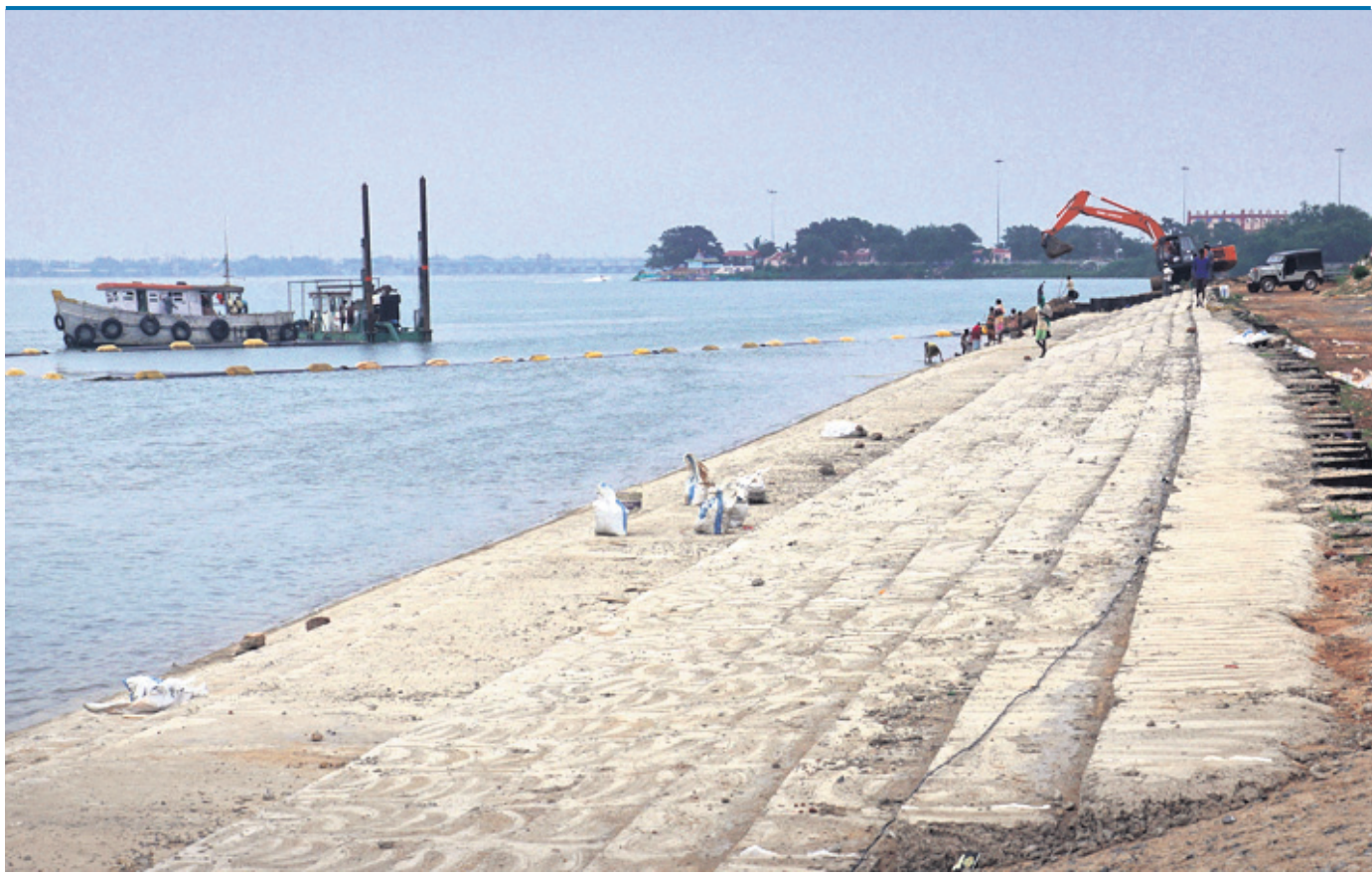
A concrete ghat is being constructed at Mahanadi river near Ballyatra ground in Cuttack, Thursday
