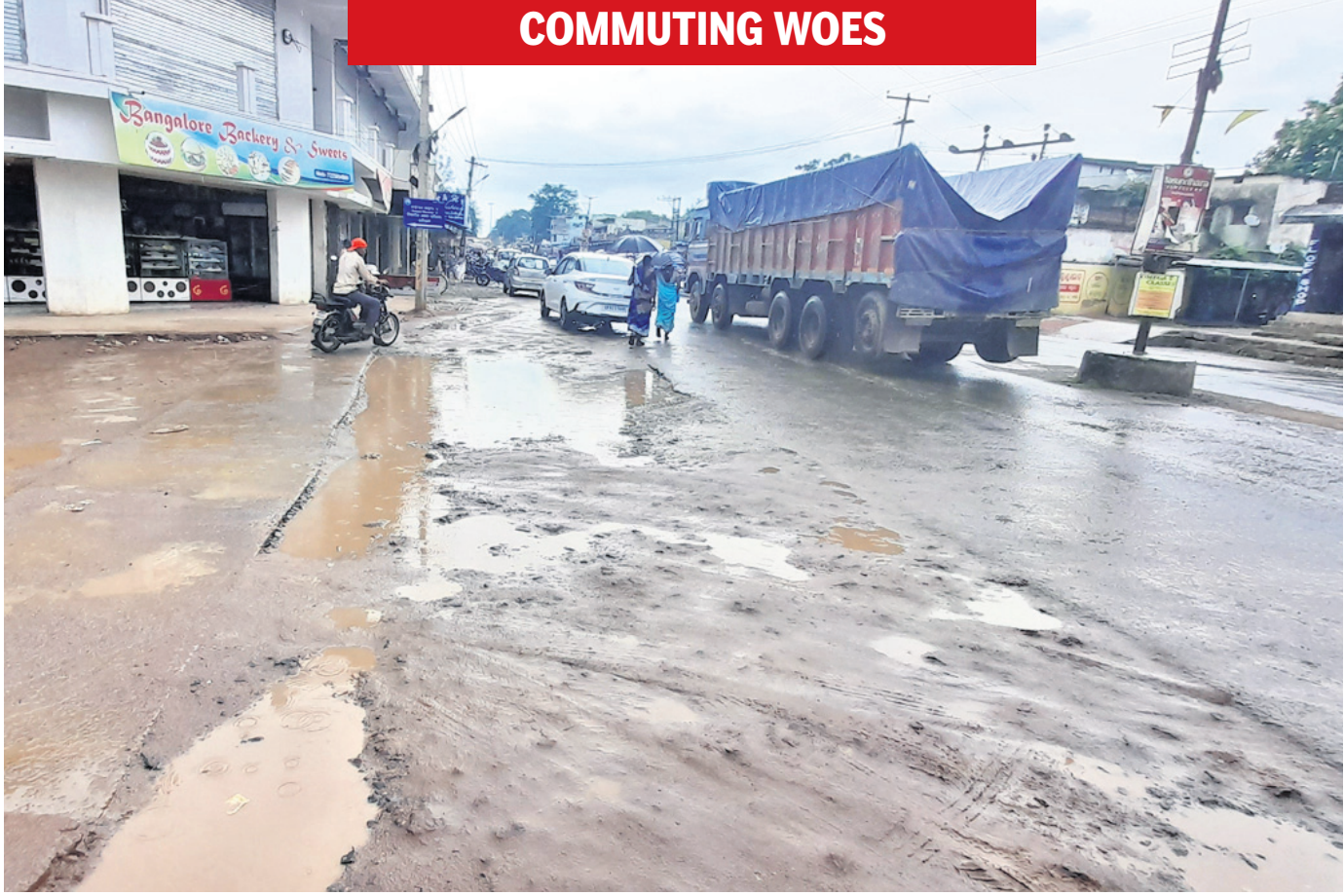
Travelling on National Highway-353 passing through Khariar town in Nuapada district has become a tough job for the commuters as craters have come up on the highway due to monsoonal rainfall
