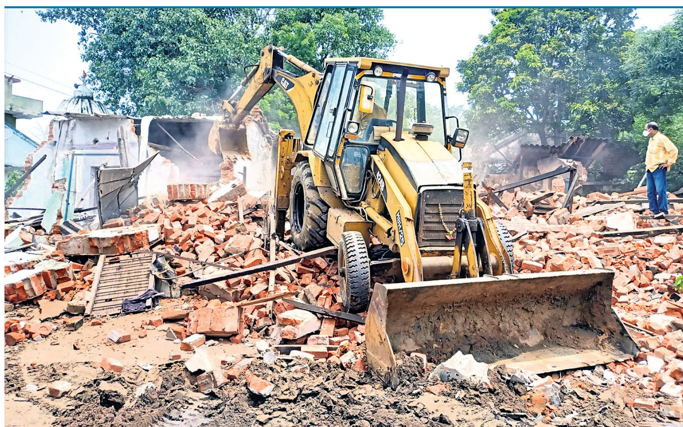
Government offices being demolished as part of an eviction drive for Samaleswari temple expansion project at Kamlī Bazaar in Sambalpur, Wednesday
