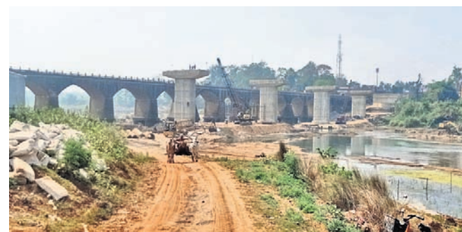
The bridge is under construction at Madhuban on the Baripada-Midnapore state highway, connecting Udala. The construction work commenced in May, 2017 and the contractor firm was asked to complete the work by December, 2018
