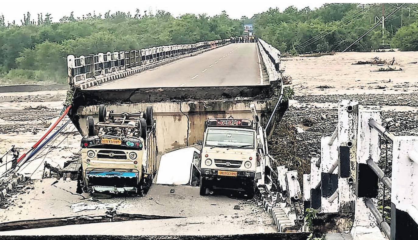
RAVAGED BY RAIN: A view of the collapsed Rani Pokhari bridge on the Dehradun-Rishikesh highway after heavy rain, near Dehradun, Friday
