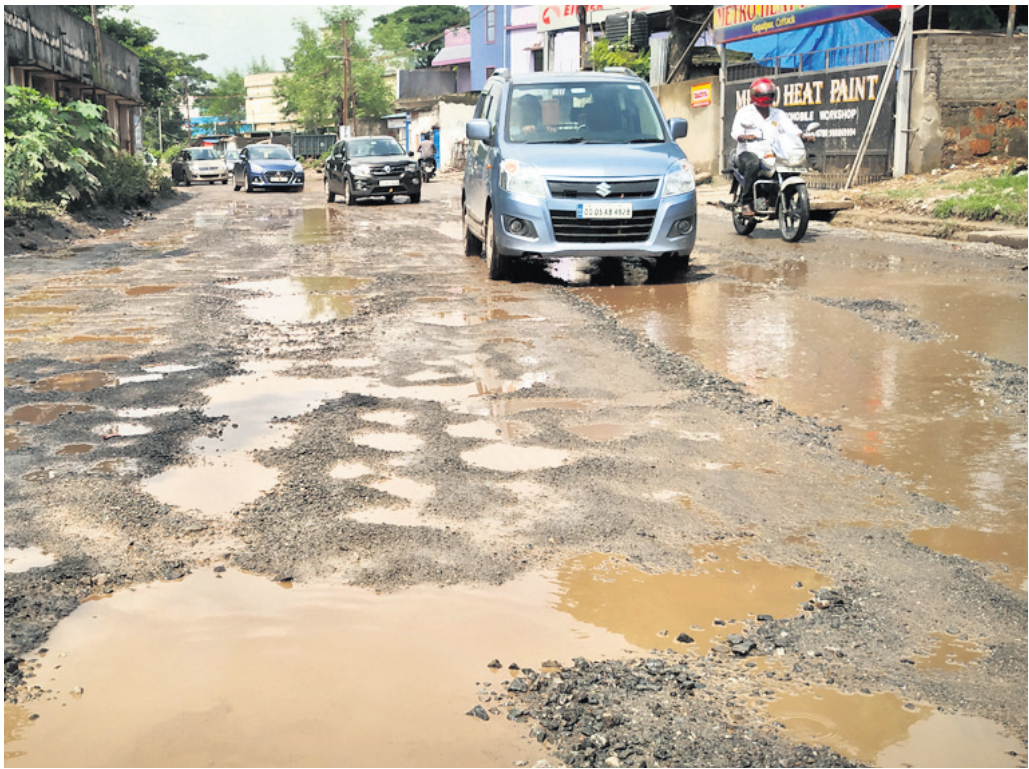
Commuters negotiating a potholed NH-16 at Gopalpur near Cuttack, Sunday
