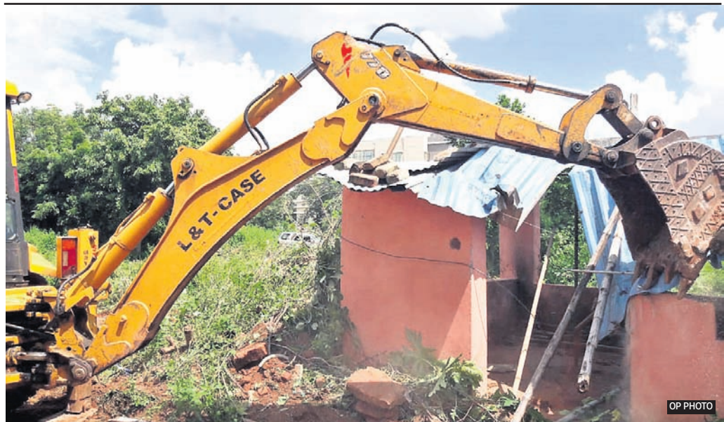
An excavator engaged by the civic authorities pulls down an illegal structure in Patia area of Bhubaneswar, Thursday
