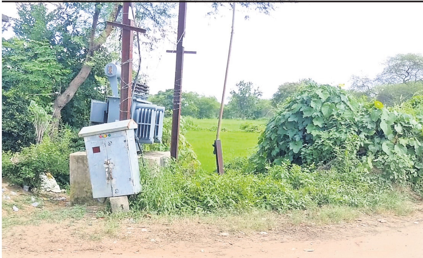
A transformer lying unprotected sans fences has endangered the lives of residents at Ghodabandha panchayat under Naria block in Kalahandi district
