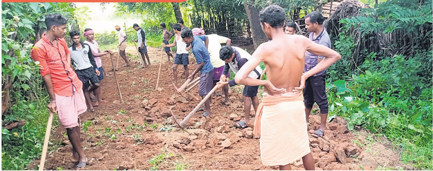
People of Kantasaru village in Kudumulguma panchayat in Malkangiri district repair a stretch of road which has been in bad shape for a long time. Villagers had drawn attention of the block administration and people's representatives towards the bad condition of the road, but nothing was done. OP PHOTO
