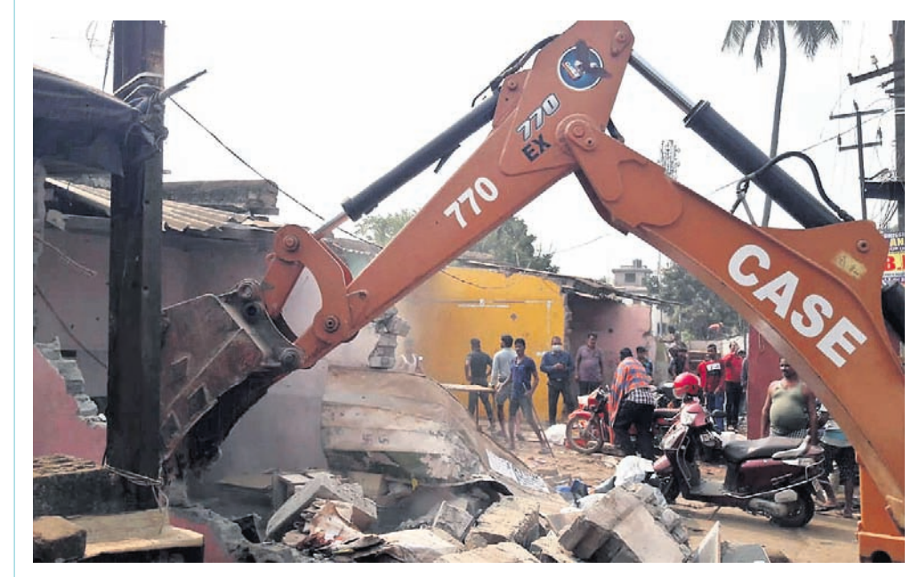
An excavator engaged by BDA pulls down structures on Bhubaneswar's Baramunda bus stand premises, Friday
