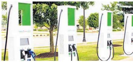
Seven more EV charging stations are likely to come up in the city in next phase
