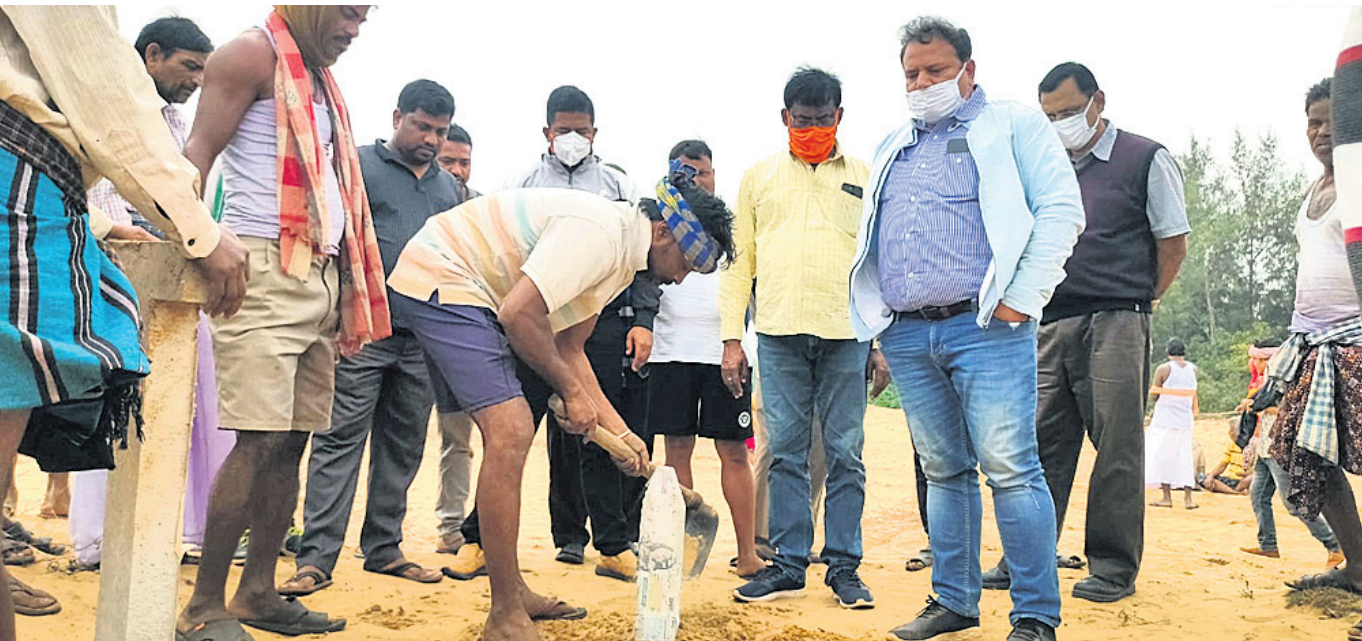
Revenue, IDCO officials and members of forest committees demarcating the boundary between newly declared revenue villages of Patana and Gobindpur under Erasama tehsil in Jagatsinghpur district for construction of a wall by IDCO for the proposed JSW project, Thursday OP PHOTO
