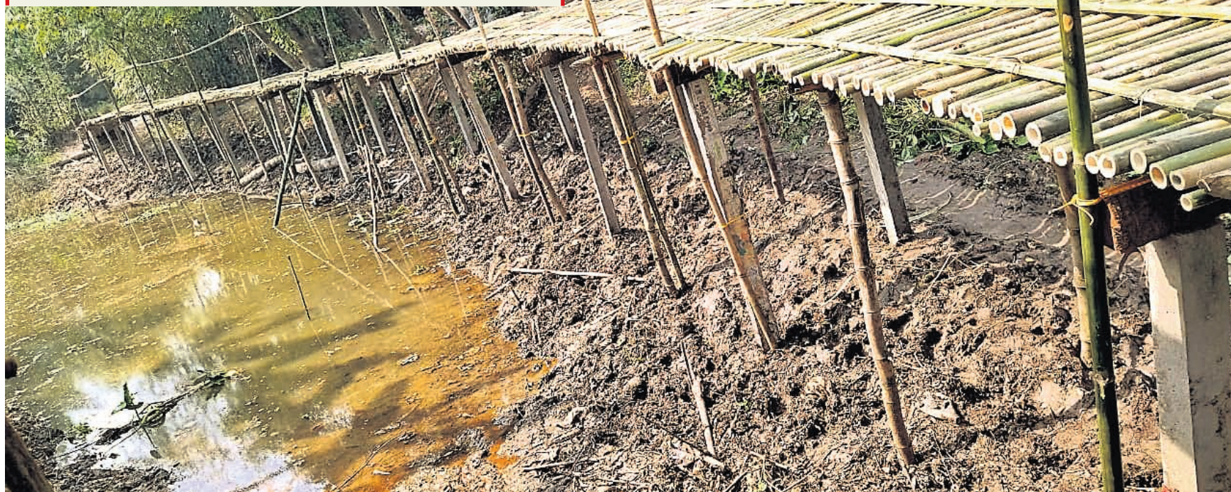
Residents of Ikda village under Khalina panchayat of Jaleswar block in Balasore have built a bamboo bridge on a 200-ft nullah to connect with the rest of the world after the administration didn't heed to their repeated pleas
