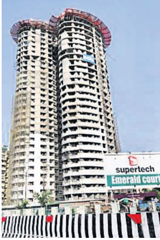
The Supreme Court Monday said the demolition work for the two 40-storied towers constructed by Supertech in Noida will begin in two weeks. PFI PHOTO
