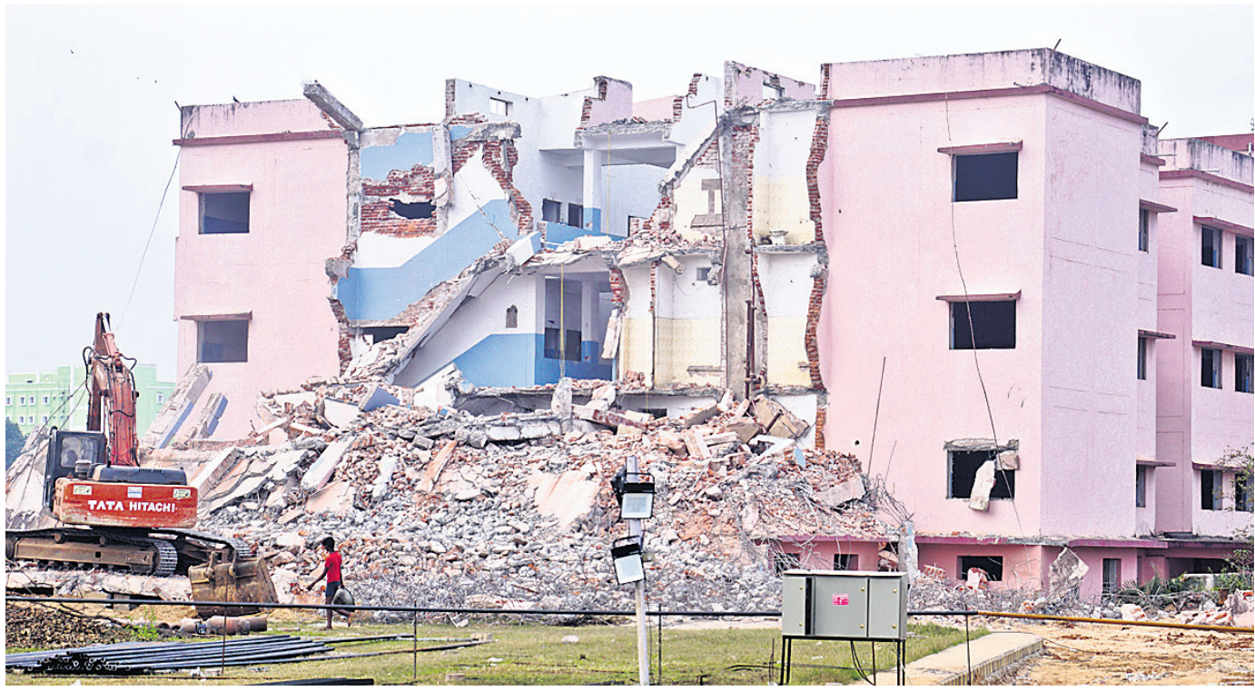
An excavator pulls down a multi-storied structure as part of the expansion of SCB Medical College and Hospital in Cuttack, Thursday
