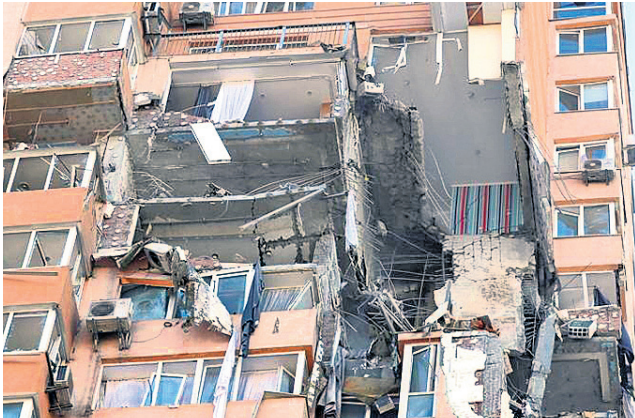
A view shows an apartment building damaged by recent shelling in Kyiv
