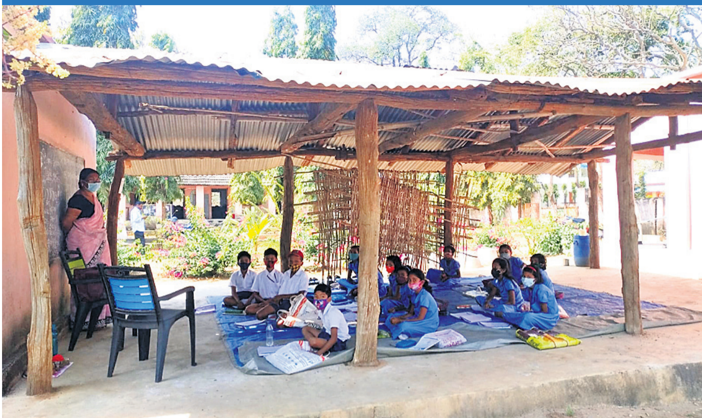
INFRA CRUNCH: Students studying under an asbestos roof at Pedipathar Primary School under Athamallik block in Angul district Wednesday
