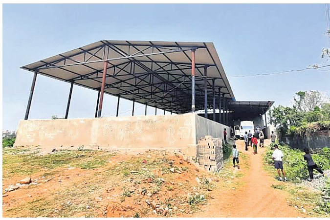
The victim's body was found from an under-construction Micro Compost Center
