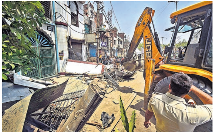
Bulldozers demolishing parts of a building in Jahangirpuri locality of New Delhi, Wednesday PTI PHOTO
