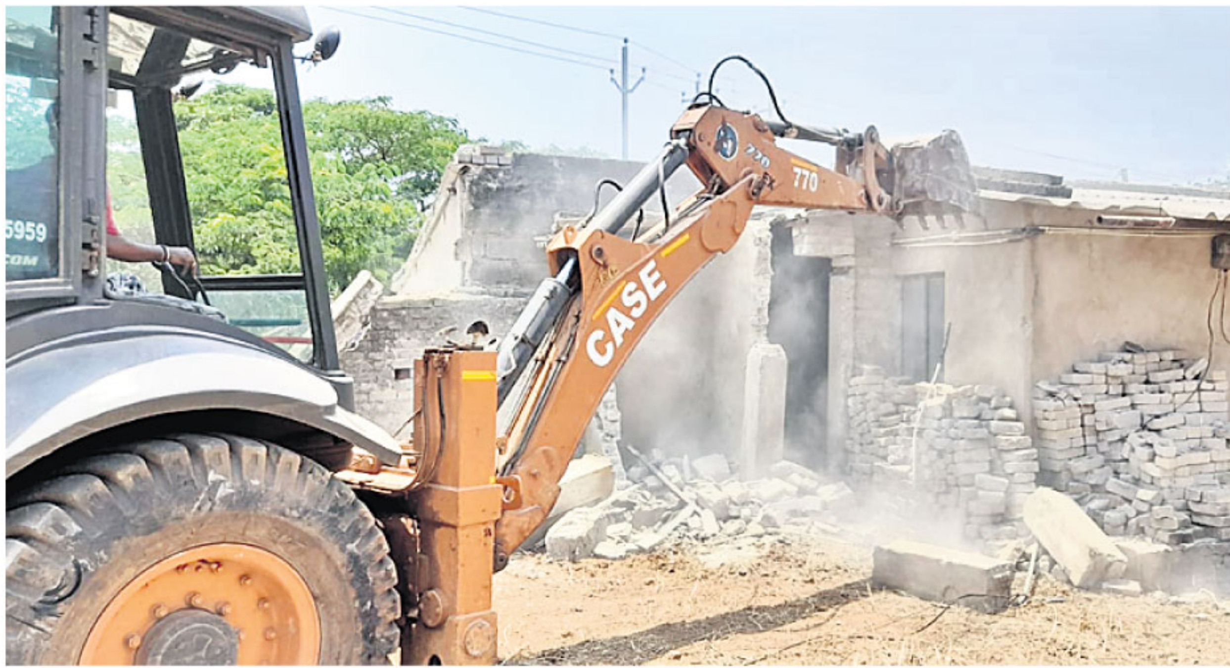
An eviction drive underway for demolition of the unauthorised constructions over a government plot in Bhubaneswar, Monday
