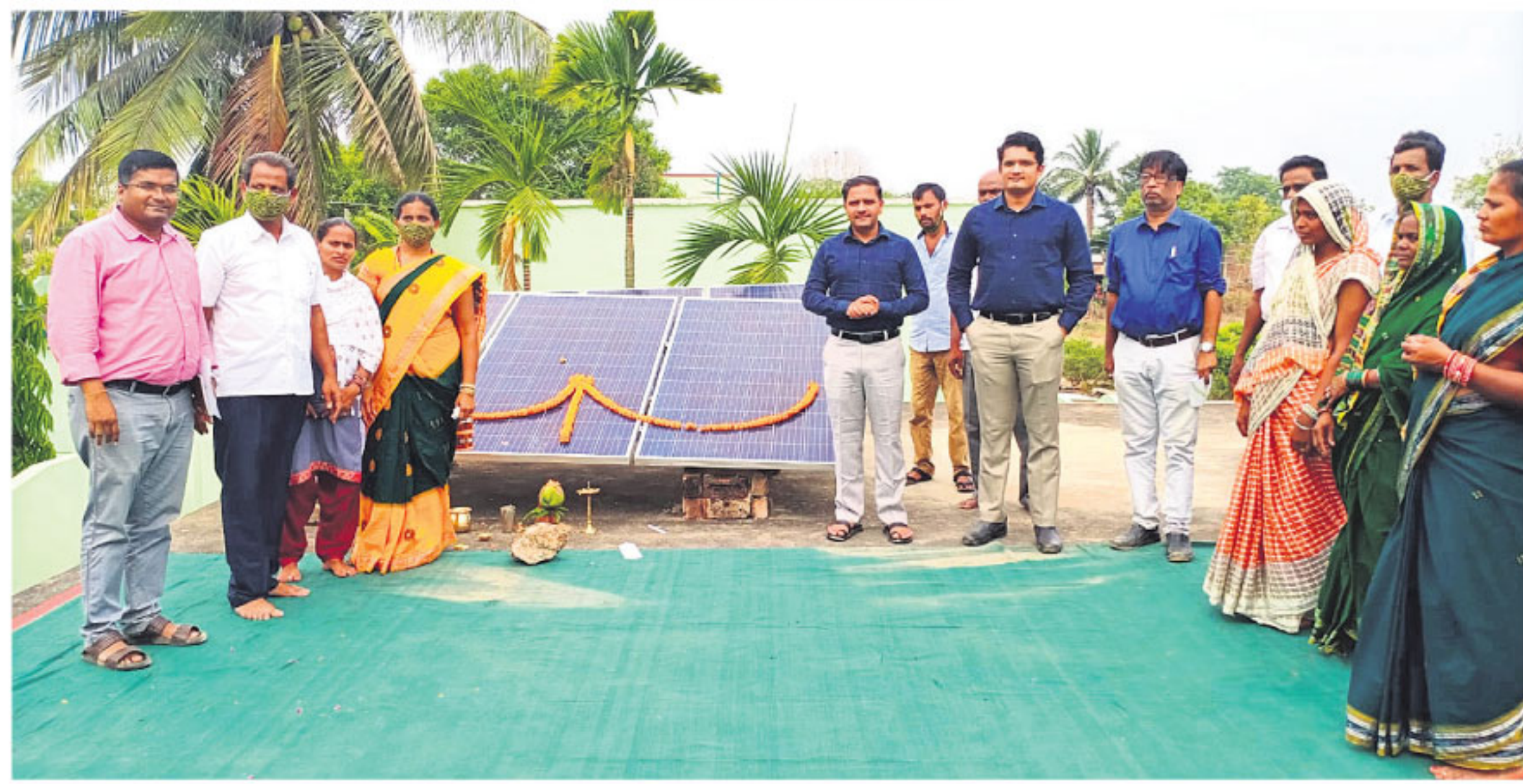
Collector Vijaya Amruta Kulange Monday inaugurated a solar plant at Pochilima High School under Hinjilicut block of Ganjam district. With this, the Pochilima and Makarjhol high schools under this block became the state's first solar-powered schools OP PHOTO
