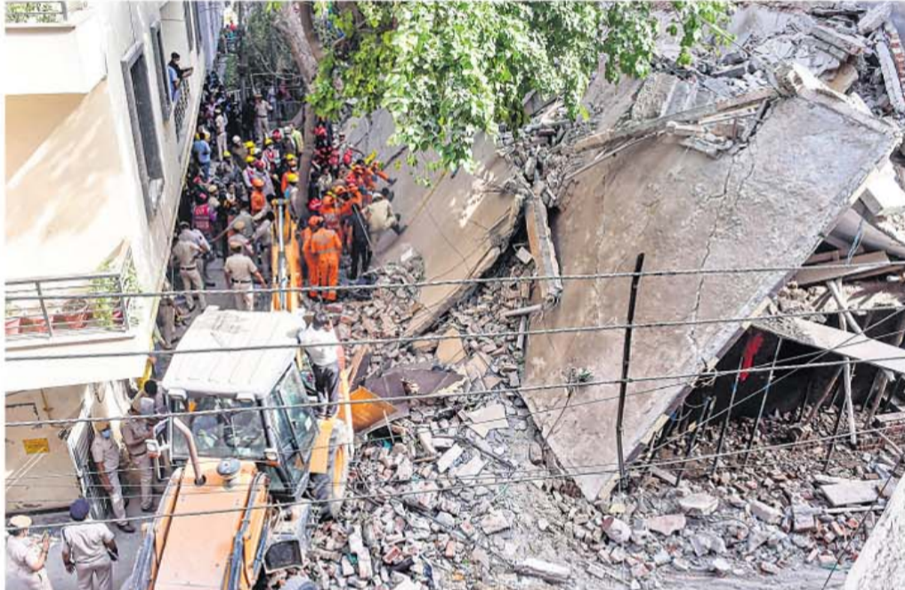
SEARCH FOR SURVIVORS: Rescue operation underway after an under-construction building collapsed at Satya Niketan area in New Delhi. Two people died while four sustained injuries in the incident
