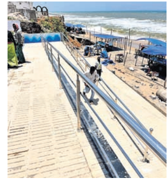
ing area to the beach. Everything from washrooms to food court will be accessible for those who use wheelchairs. Moreover, the food counters will be at a lower height
