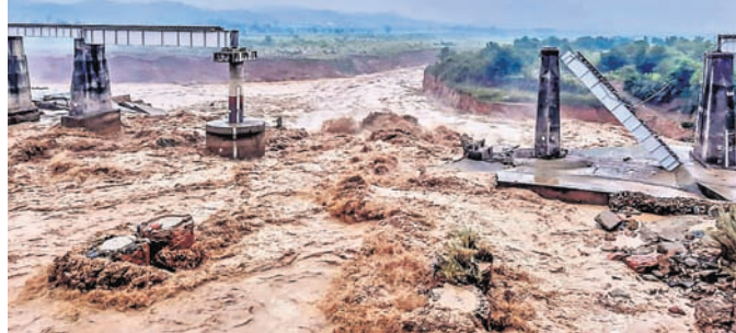
Collapsed portion of a railway bridge over Chakki river in Himachal Pradesh
