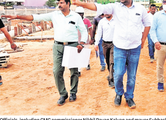
Officials, including CMC commissioner Nikhil Pavan Kalyan and mayor Subhash Singh, take stock of Netaji Bus Terminal construction in Cuttack, Saturday
