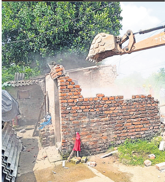
An excavator deployed by BDA demolished illegal structures at Mahishakhala in Bhubaneswar, Thursday
