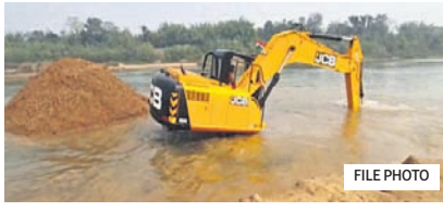
environmentalist-cum-honorary wildlife warden Bibekananda Pattanik filed a complaint before the National Green Tribunal. The NGT admitted the petition (Case no-46/22) for hearing and heard it April 22, 2022. During the hearing, it directed the Mayurbhanj district collector to file its reply by April 26. The petitioner alleged that the report prepared on minor mineral management is an interim one and the officials concerned have not visited the areas required to for the survey.
