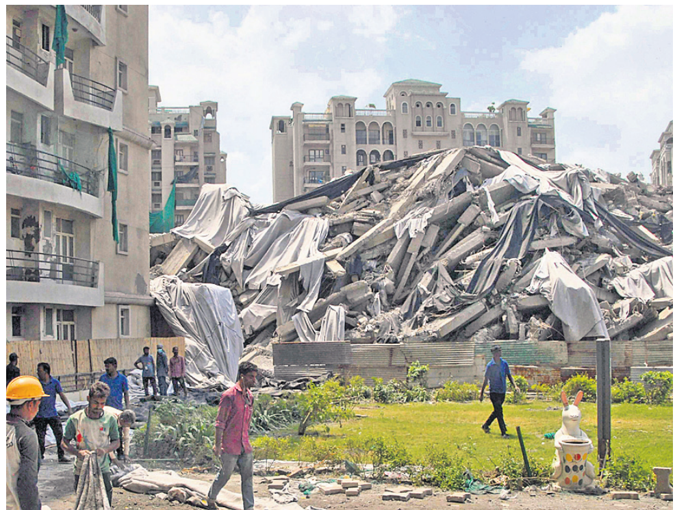
Workers clear debris near the site of the demolished twin towers of Supertech, in Noida, Wednesday. Over 3,700 kg of explosives were used to bring down the two towers by waterfall implosion technique leaving approximately 80,000 tonnes of debris.
