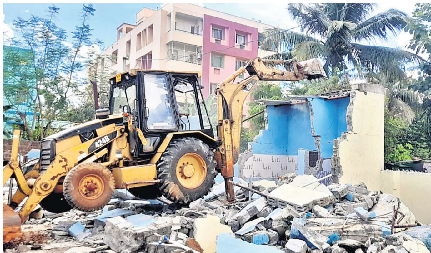
An excavator engaged by the civic body pulls down an illegal structure in Chandrasekharpur area of Bhubaneswar, Friday
