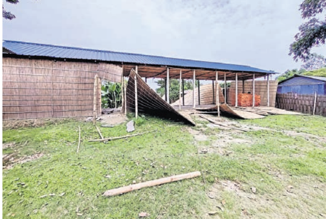
The demolished madrasa at Darogar Alga village in Goalpara district PTI PHOTO
