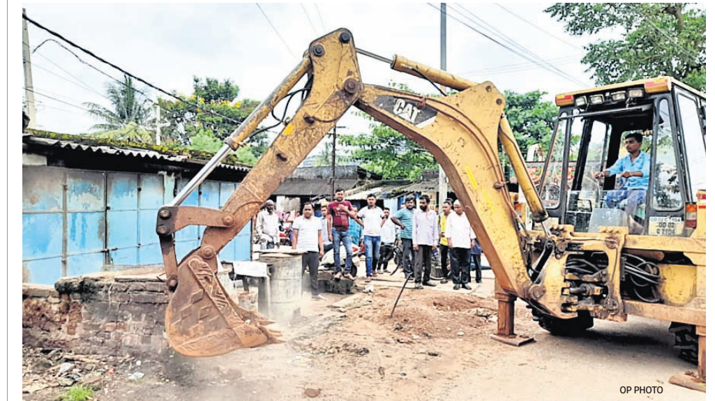
An excavator deployed by BDA razing down an illegal structure in Chakeisiani area of Bhubaneswar, Monday
