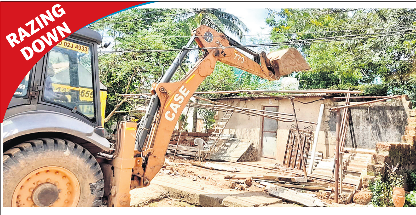
An excavator deployed by BDA razing down an illegal structure at Aiginia in Bhubaneswar, Thursday
